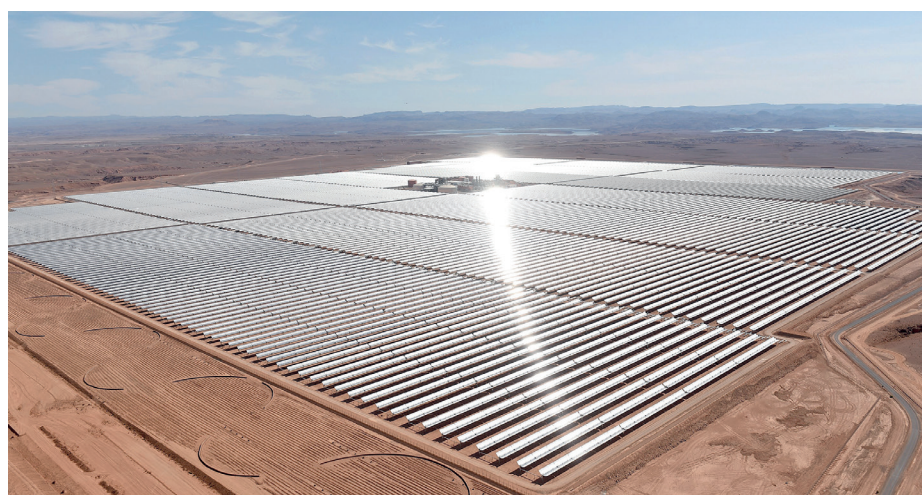
The Noor Ouarzazate complex is the first solar project developed as part of the Moroccan energy strategy which aims to increase the share of renewable energies in the national electricity mix to more than 52% by 2030
