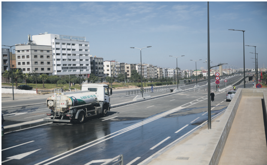
The bridge is open to traffic, while work continues below the bridge for the creation of the largest interchange hub in the public transport network on its own site, which will bring together the services of Line 3 of the tram and BW1 near bus and large taxis stops
