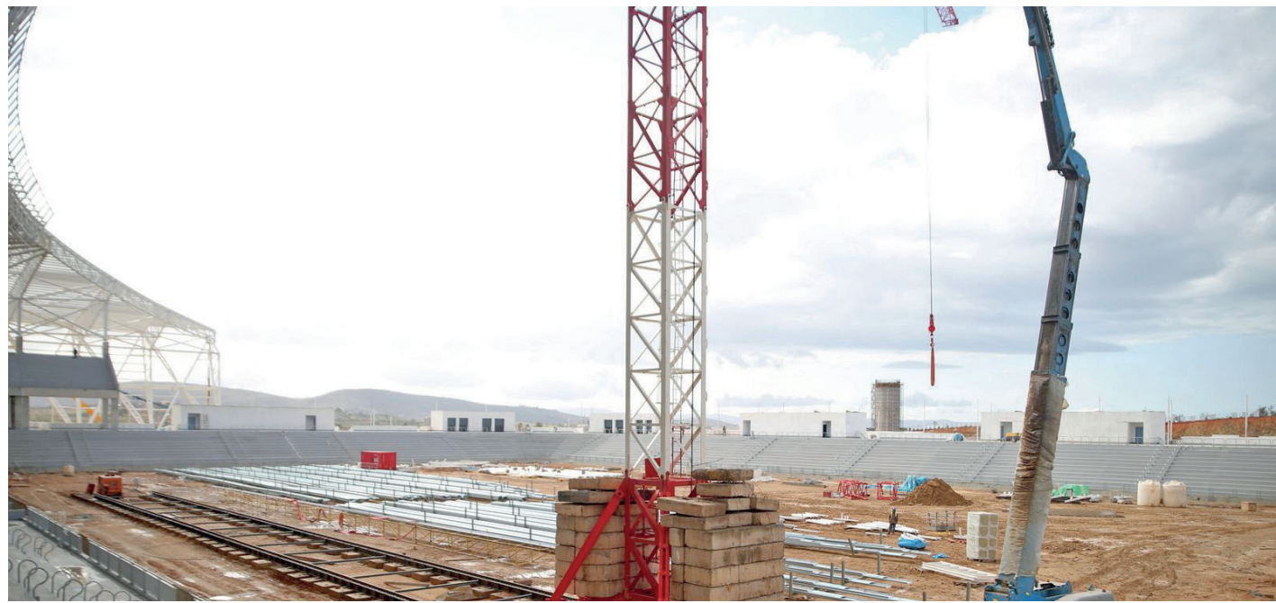
The reform proposes to introduce the national call for tenders as a new procedure, reserved for Moroccan companies, with a ceiling depending on the type of work (works, supplies, and services) ( Ph. L'Economiste)
